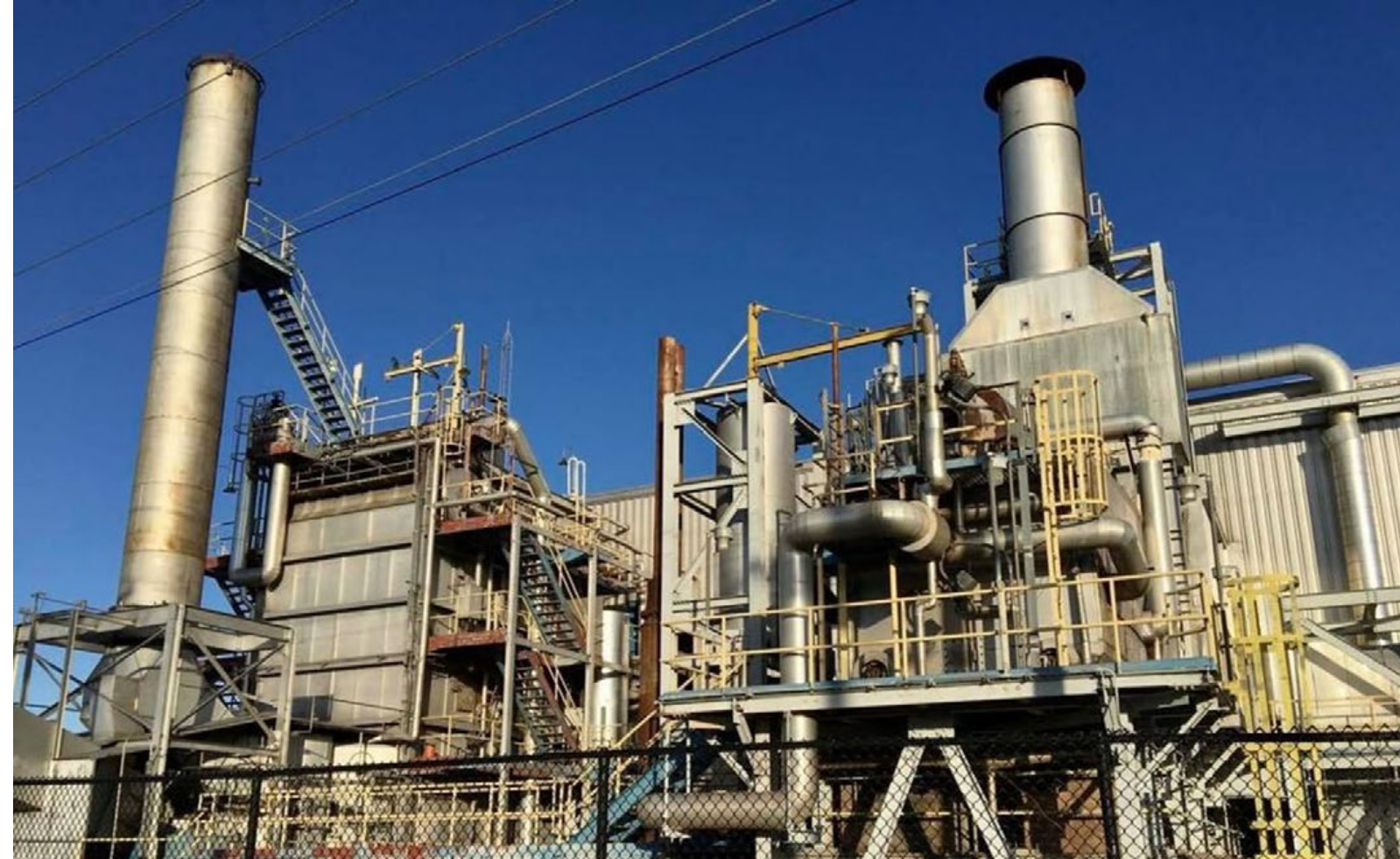
Boomer Lake Station – Lakeview Landing in Stillwater, OK
