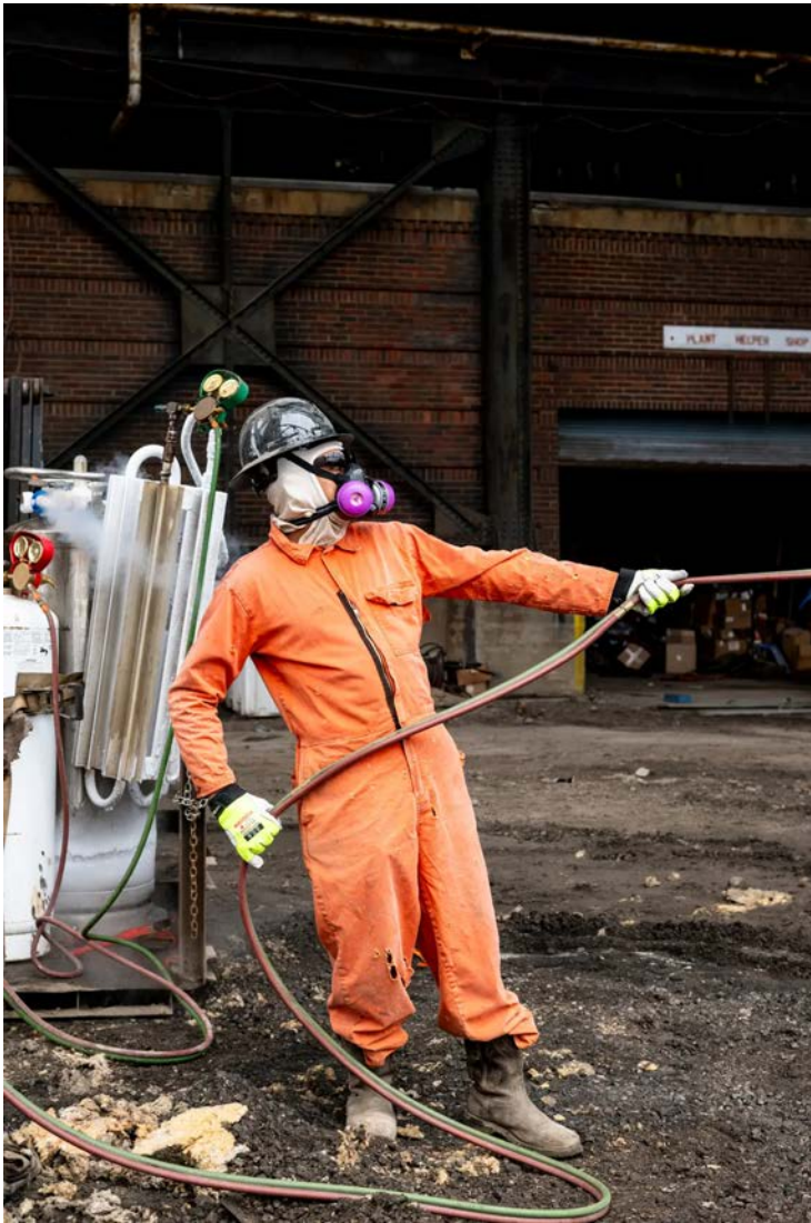
A member of the demolition crew at the plant . . . Daniel Lozada for The New York Times
