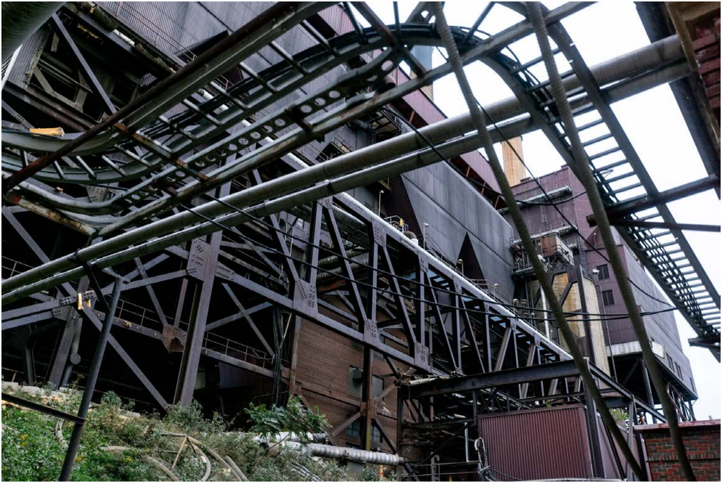
Redevelopment of the power plant offers a chance to create public access to the Lake Erie waterfront. Daniel Lozada for The New York Times
