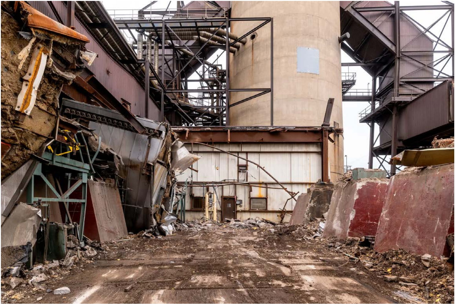
Workers removed 3,000 tons of asbestos, shipped out 36,000 tons of unused coal and extracted 140 tons of steel from demolished buildings. Daniel Lozada for The New York Times
